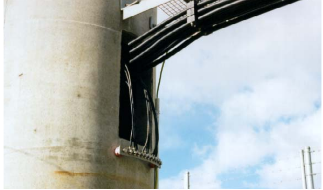
Figure 9. Cable sheath bonding at the base of the tower
